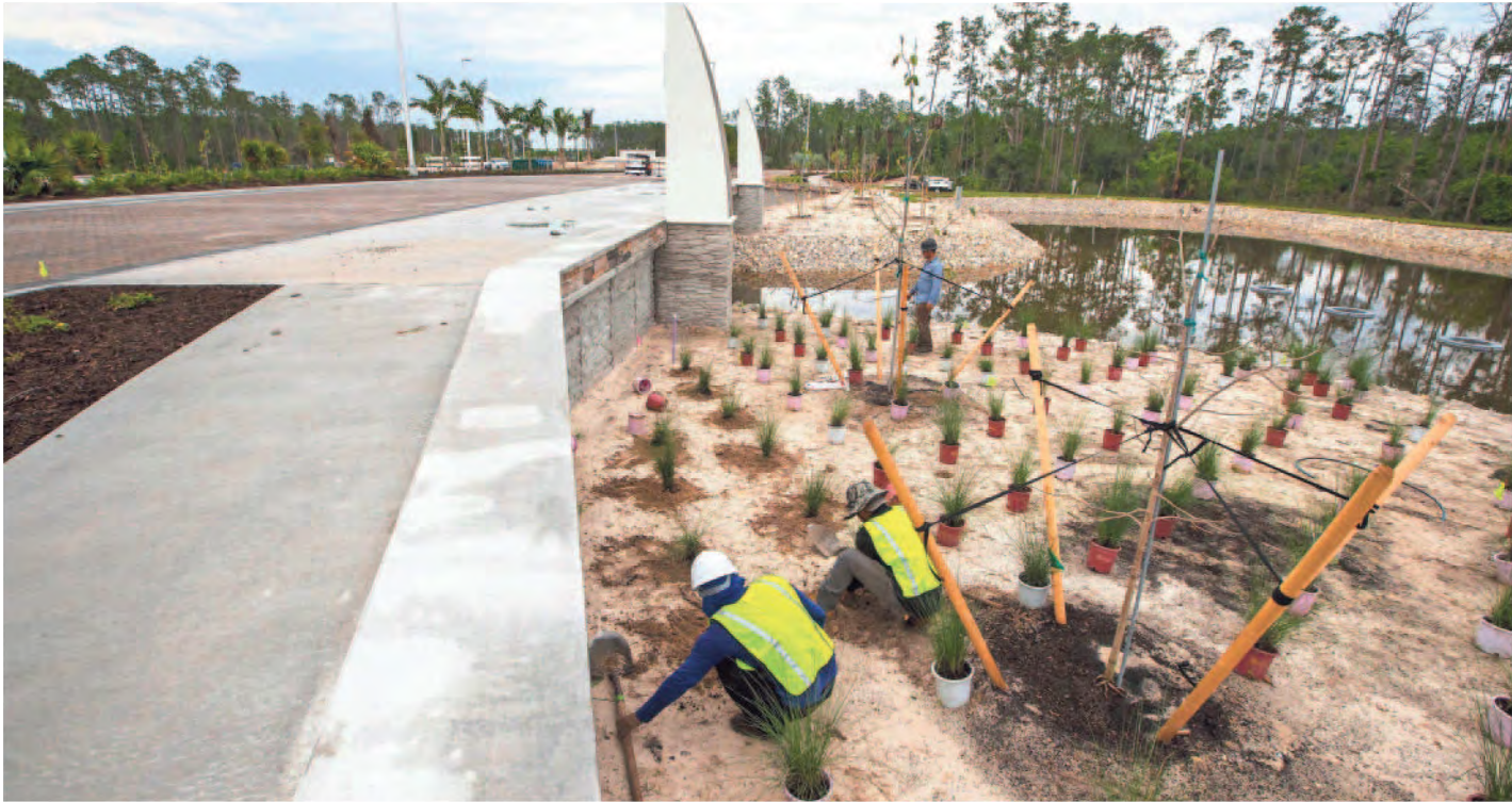
Work continues at an entrance point to the new Skyplex commercial development. RICARDO ROLON/THE NEWS-PRESS
