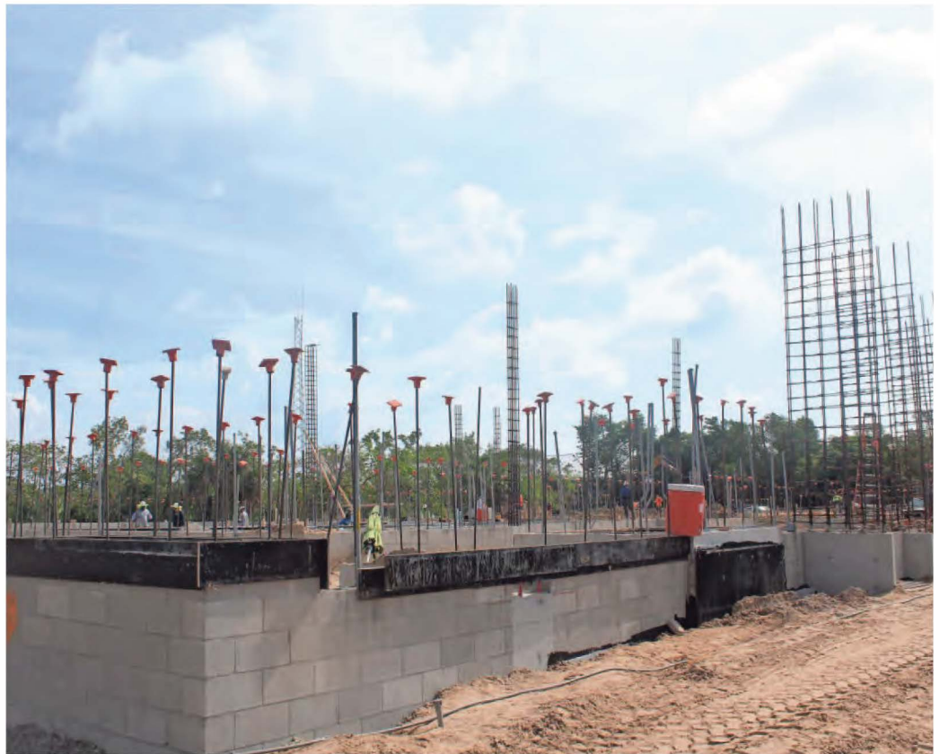
Big Arts is under construction at the same site of its previous building on Sanibel Island. SPECIAL TO THE NEWS-PRESS
