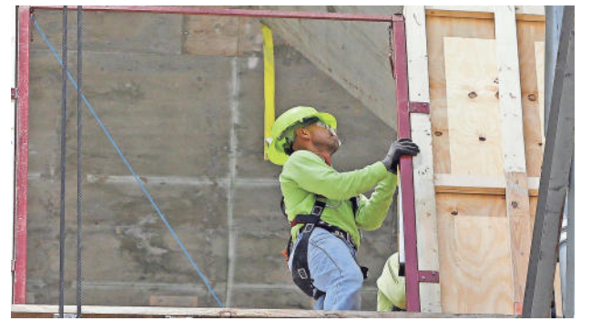
ALAN DIAZ/AP A construction worker works on a high-rise condominium project in downtown Miami.
